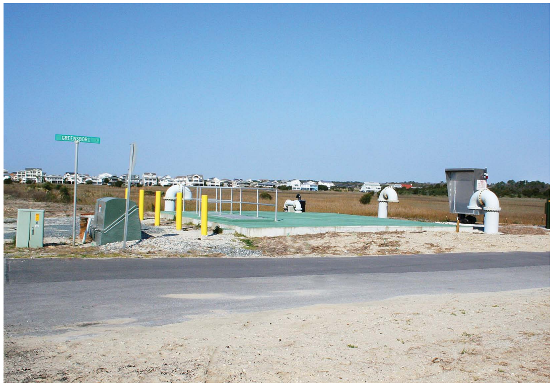
Holden Beach had its four vacuum stations built below grade in watertight vaults, which provides an aesthetic benefit and protects the system from storm surges.
