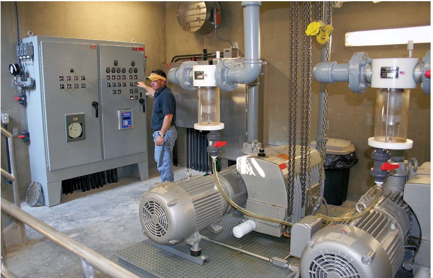
Vacuum stations provide a clean, safe environment for system operation and monitoring.
