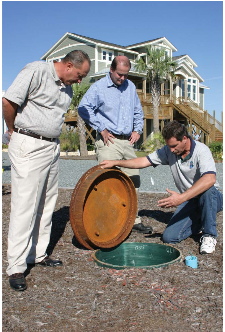
Frank Bland, AIRVAC regional manager (left), and Bart Sanders, AIRVAC field representative (right), explain how a vacuum valve pit works to Steve Wheeler, Holden Beach town manager (center).
