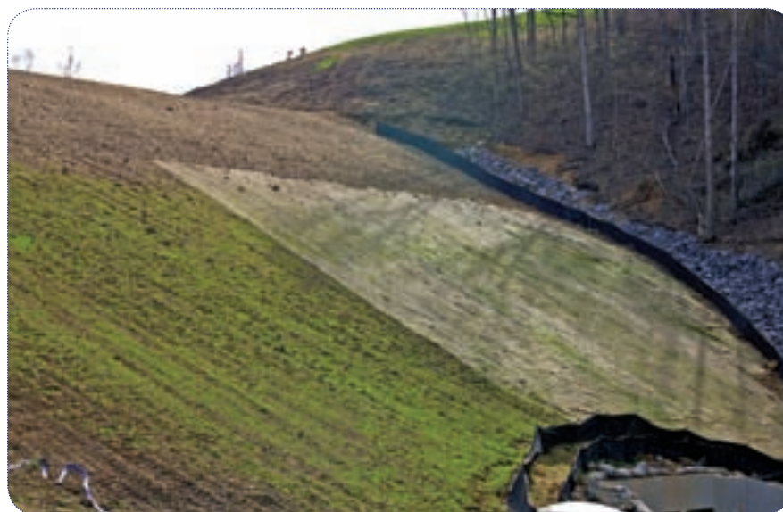
ALDOT tested various products, including blown straw and a single net straw erosion control blanket, on the I-22/I-65 site.
