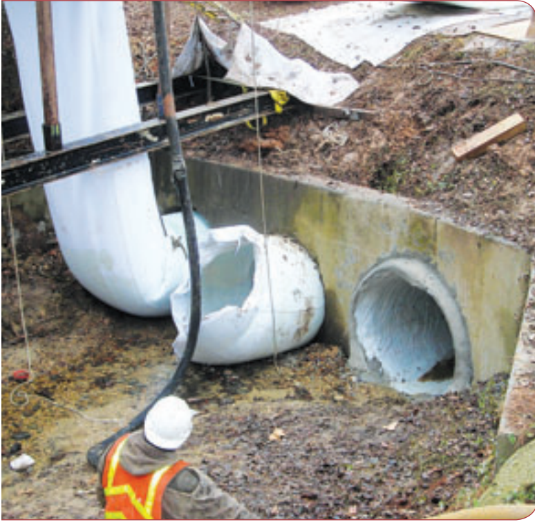
The county converted from open-cut methods, piggybacking on an existing CIPP contract.
