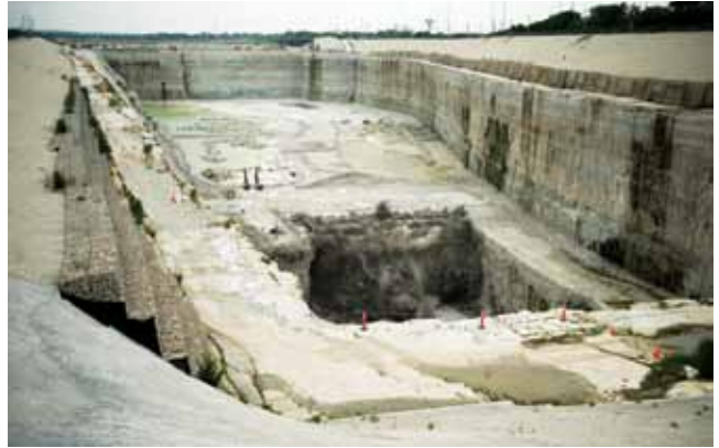
In September 2013, the final blasting took place on the Thornton Composite Reservoir, which is scheduled for completion in 2015.
