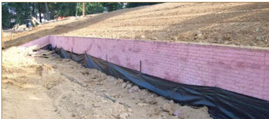
Retaining walls helped minimize the footprint of the CBU soccer field while maintaining the basin's required water retention level.
