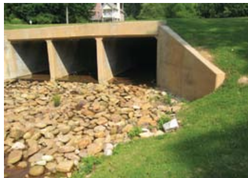
The WSA showed customers how storm water fees improve the community. For example, storm water infrastructure before (far left) and after (left).
