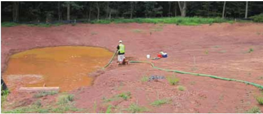
Once the water began to exit the system, approximately five complete evacuations of the chambers were completed.
