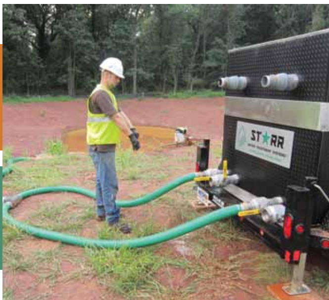
Hoses were attached to influent valves on the system and placed into the sediment pond.
